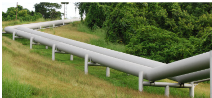
The SOTE pipeline, pictured above, was one of the two major Ecuadorean oil pipelines that ruptured last month. // File Photo: Ecuadorean Government.
