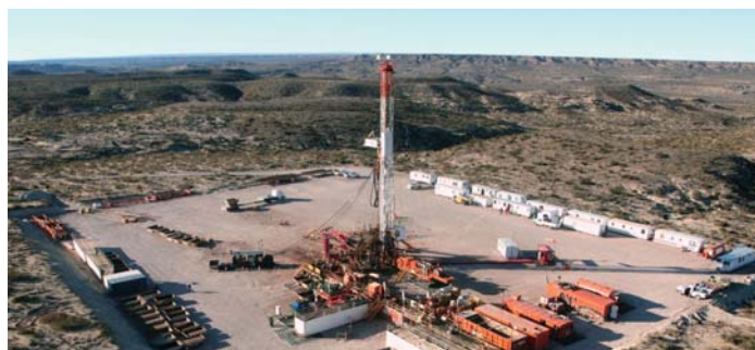
A drilling pad in the Rincón del Mangrullo block, one of Argentina's leading unconventional gas developments. // File Photo: BBVA.
