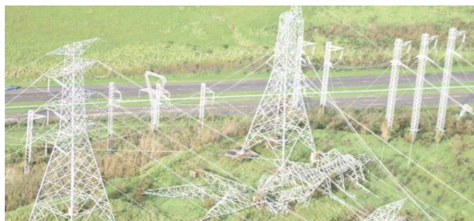
Hurricane Maria left serious damage across the Caribbean, including downed power transmission infrastructure in Puerto Rico. // Photo: Commonwealth of Puerto Rico.
